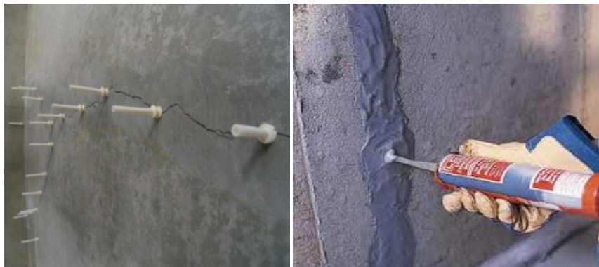
Fig 1: Injection of epoxy bonding compounds or non-shrink cement grouting under pressure Repair / Rehab
